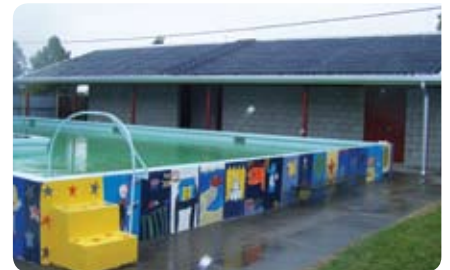
Sefton school's pool in Canterbury, alongside the solar heating system sits above the changing sheds.
